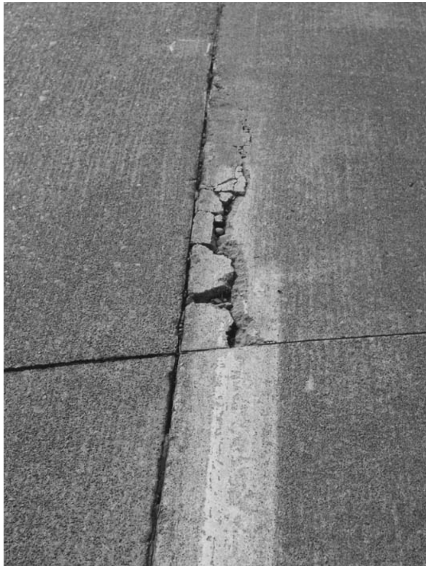
Figure 11. A typical location for a spall is along a joint, usually the result of the joint functioning improperly. (67216)
