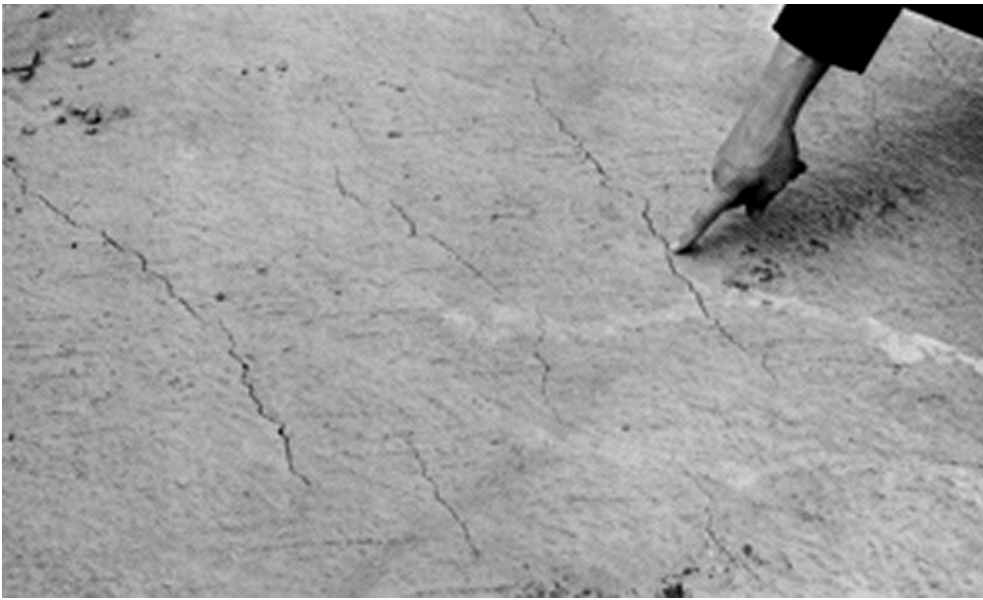
Figure 2. Plastic-shrinkage cracks caused by rapid loss of mix water while the concrete is still plastic. (1311)
